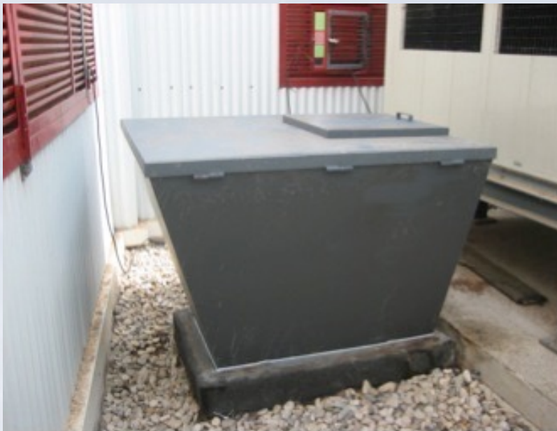
Biomass hopper tank
